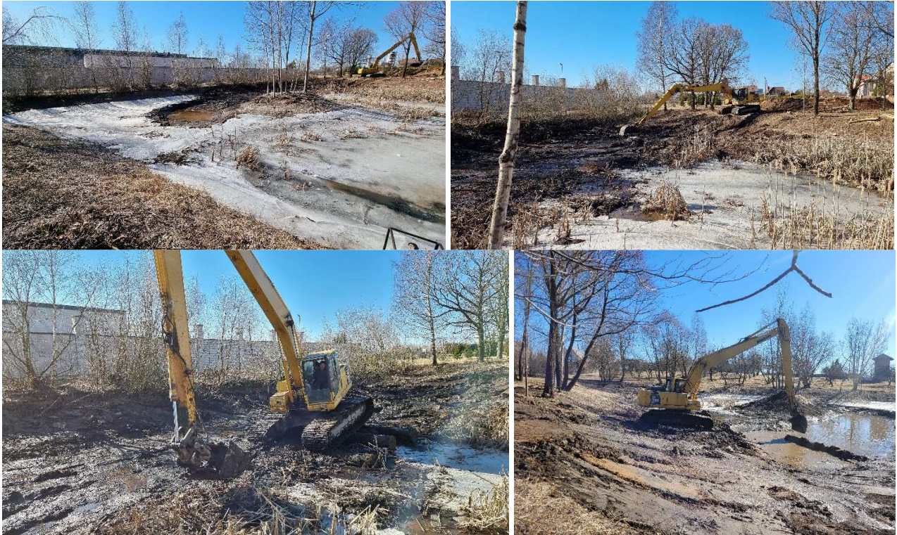
Figures 45, 46, 47 un 48. Cleaning and deepening of the Anykščiai Green pond (Photo: A. Balevičius and E. Abramovaitė)
